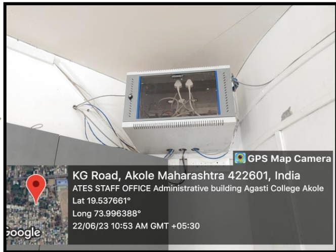
Networking Components Rack, ATEs Office
